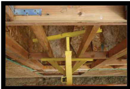
4. Jack is ready for planks first then handrails. All three 2x4 handrails must be installed and secured with 8 penny nails. Handrails can be installed in outer pocket to allow three standard OSHA scaffold planks or the second pocket to accommodate two plank applications. Check your OSHA regulations for allowable spacing between wall and first plank.
