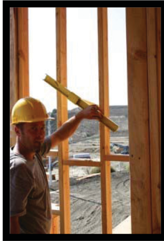
2. Check that studs have been properly attached to bottom and top plate.
